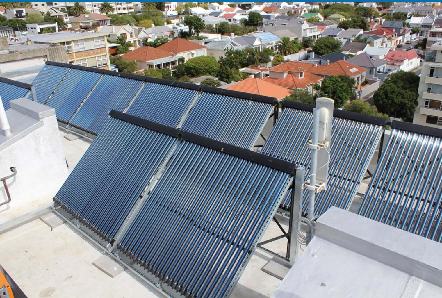
85 m² evacuated tubes at Centurion Building, CapeTown
