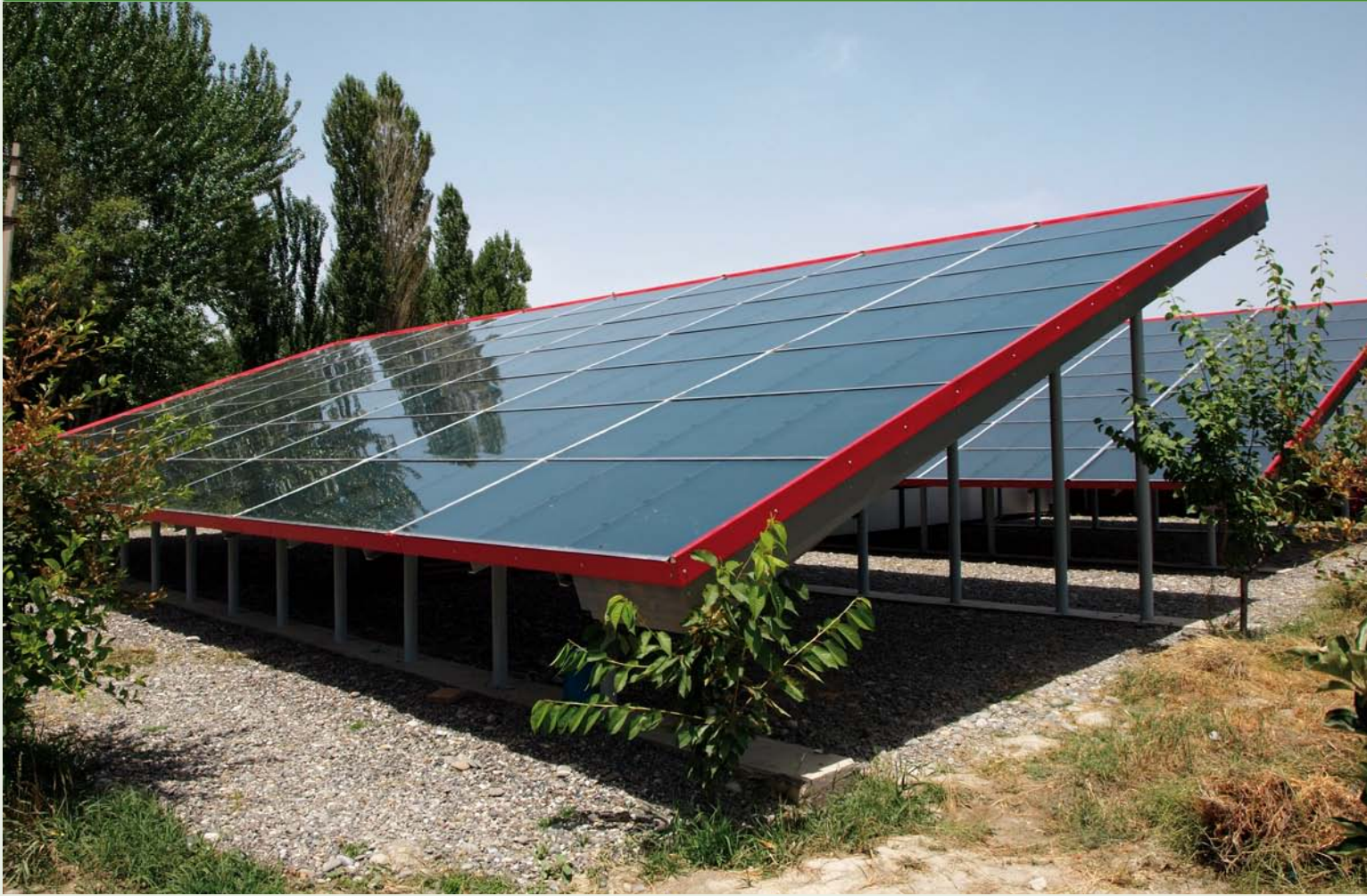
Solar air collector system in Uzbekistan.
